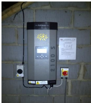
Picture showing the Inverter installed. Safety notices and Isolators.
