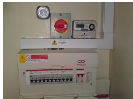
Picture showing the Consumer unit, Main Isolator and PV Meter. Another tidy job!
