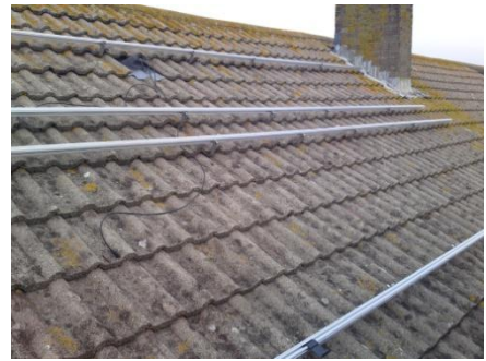
Picture showing the finished rails and cable entry. (Now ready for the panels)
