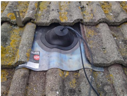
Picture showing method of cable entry. (This is eventually behind the panels).
