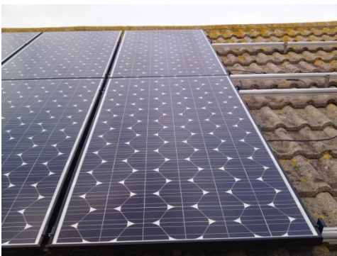
Picture showing the fixing of the Panels to the rails. (These are Sanyo HIT 240)
