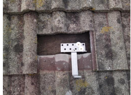
Picture showing the roof anchor being fixed to the common rafter (Truss).
