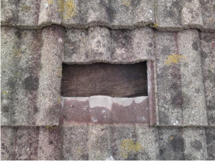
Picture showing the tile being pushed up.
