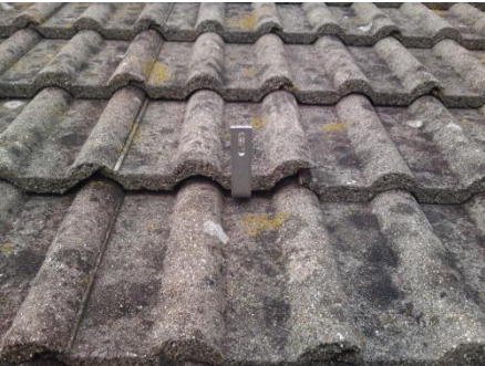
Picture showing the finished look of the tiles after the roof anchor has been installed.
