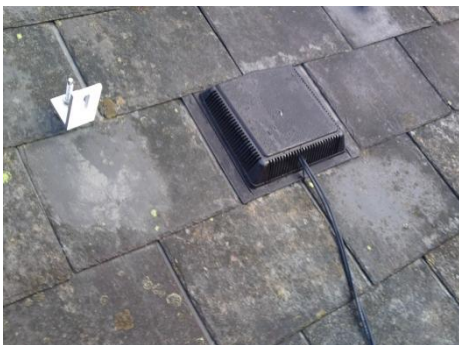
Picture showing method of cable entry. (This is eventually behind the panels).
