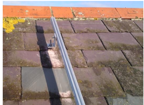
Picture showing the rails mounted vertically on the roof anchors.
