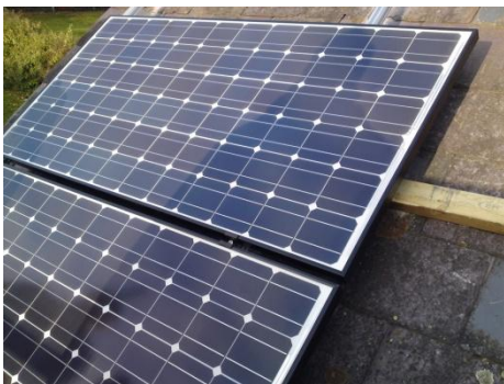
Picture showing the fixing of the Panels to the rails. (These are Sanyo HIP 215)
