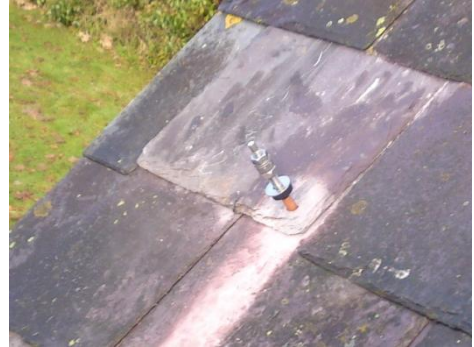
Picture showing the roof Bolt being fixed to the common rafter (Truss).
